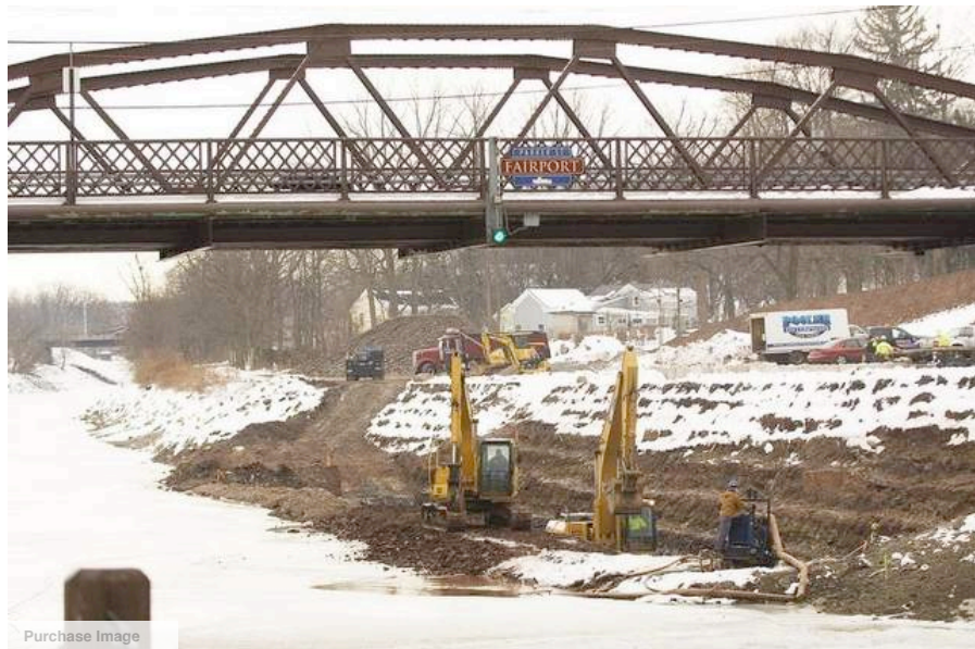
Crews begin work to construct a cement retaining wall on the Erie Canal in the village of Fairport that will allow boats to dock along a new public promenade just east of the Parker Street bridge. / Jeffrey Blackwell//Staff Photographer
